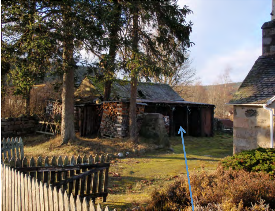
Shed to be replaced
